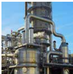
Pipe still furnaces
